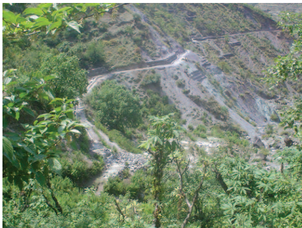
Photo 1: Roads are built in three different phases. Often traditional trails are widened to tracks and roads.
