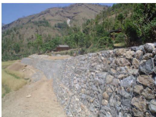
Photo 3: A gabion structure fortifies the lower side of the road, where the soil and groundwater is soft and heavy rain-falls cause erosion
